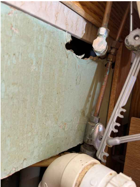
Bathroom 3 Sink Valves
