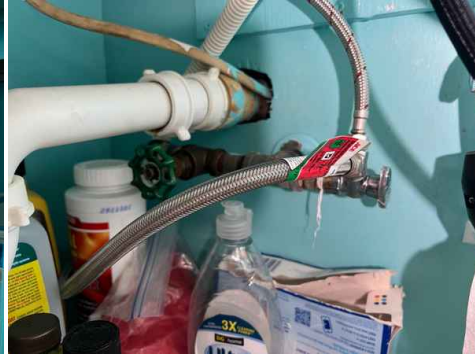
Kitchen Sink Valves
