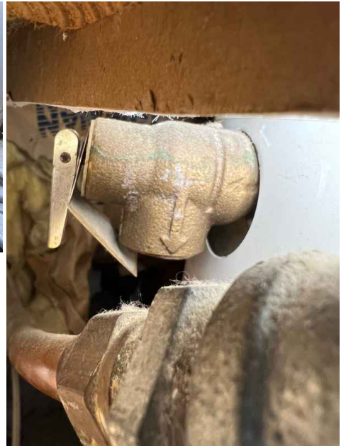
Water Heater 2 TPR Valve
