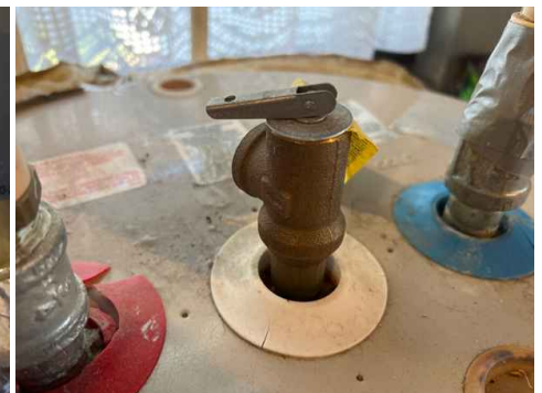
Water Heater 1 TPR Valve
