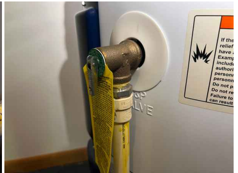
Water Heater 3 TPR Valve
