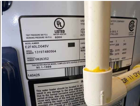
Water Heater 3 Label
