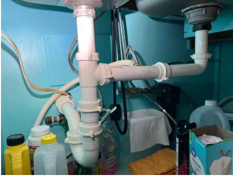
Kitchen Sink Drain
