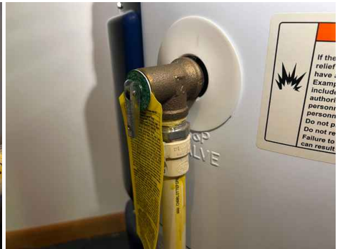
Water Heater 3 TPR Valve
