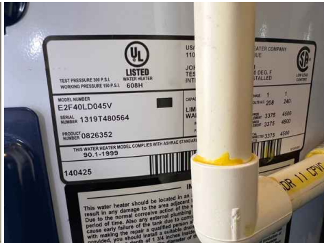
Water Heater 3 Label
