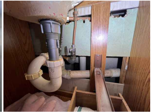
Bathroom 3 Sink Drain
