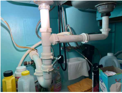
Kitchen Sink Drain
