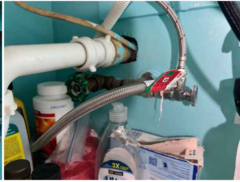
Kitchen Sink Valves
