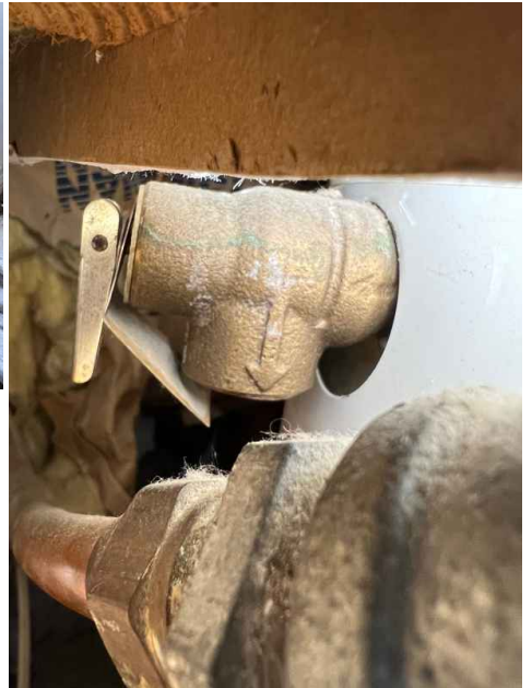
Water Heater 2 TPR Valve
