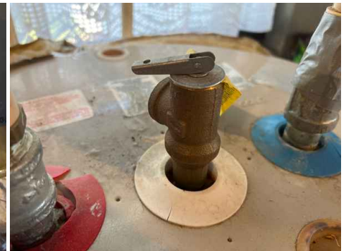
Water Heater 1 TPR Valve
